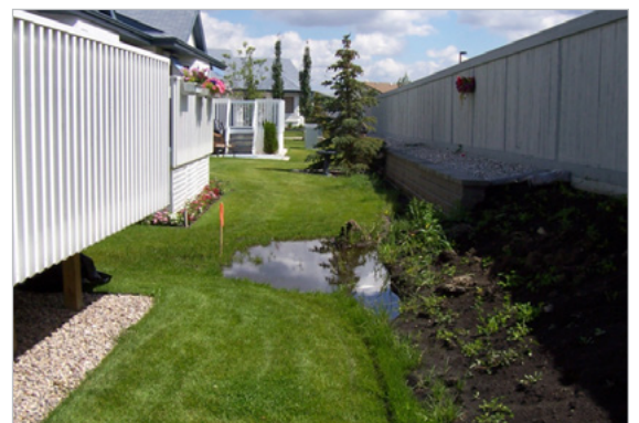
Poor grading in this drainage swale causes water pooling
