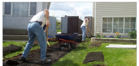
An internal drainage swale being built using a string-line as a visual guide for the slope of the swale
