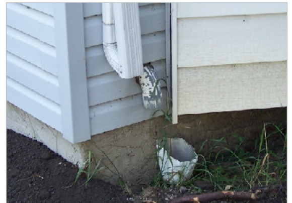
Downspout disconnected from storm service
