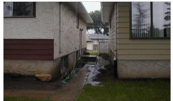
Locations with poor lot grading generate a risk of basement flooding during rain events
