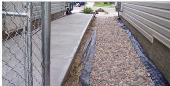
This new sidewalk does not have 15 cm drainage space within the property.
