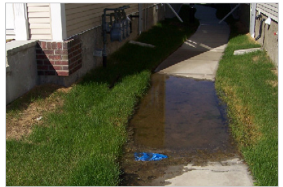
Sidewalk settlement between two condominium units results in pooling of water
