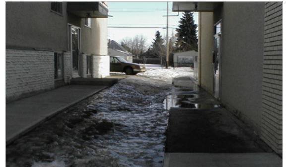
Poor lot grading between two apartments creates a low area for ponding during snow melt
