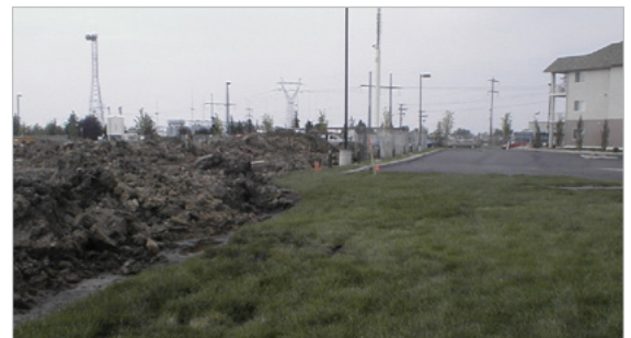
This new apartment site is in violation of the bylaw because it has the surface runoff flowing towards the abutting lot.
