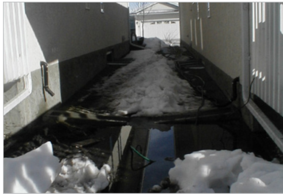
Poor lot grading results in flooding between two condominium units
