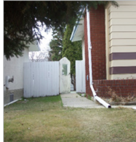
With a slope towards the foundation on the left, stormwater will flow towards the left house.
