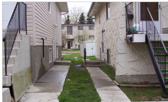
The sump pump discharge on the left drains towards the right property, which has a slope towards the foundation wall.
