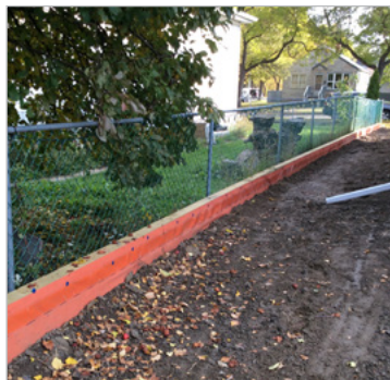
Example of internal swale and retaining wall at rough grade with dimpled waterproof membrane
