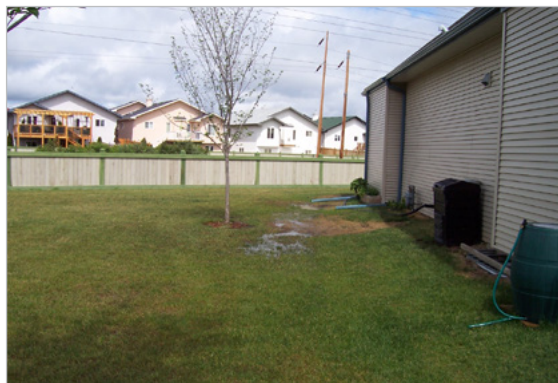
Settlement beside this condominium unit causes water pooling and potential basement flooding
