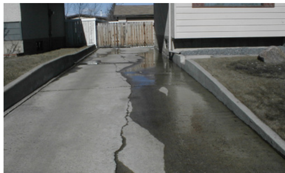
Property on right with negative grade and evidence of surface runoff at foundation wall
