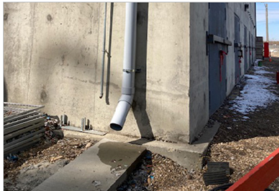
Example of downspout with a concrete splash pad at an industrial building
