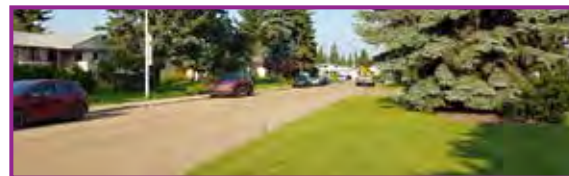
Missing sidewalk along the south side of 131A Avenue between 123A Street and 123 Street.
