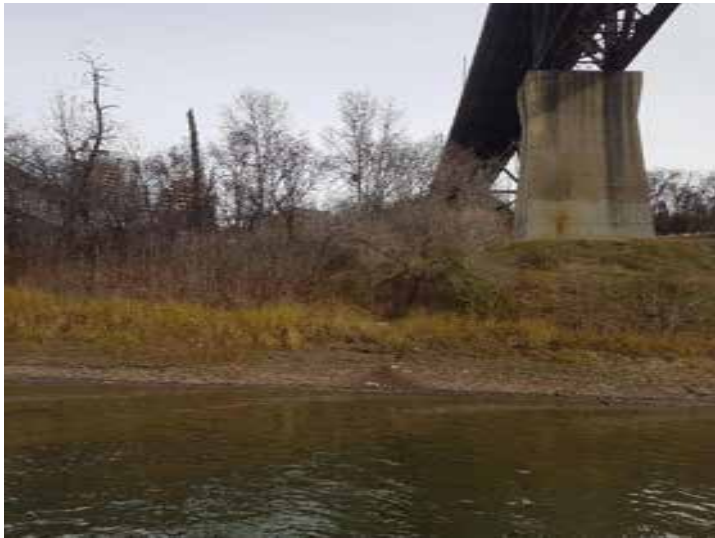
Plate 31: Looking at the north end of the High Level Bridge between Transect 16 and Transect 17.
