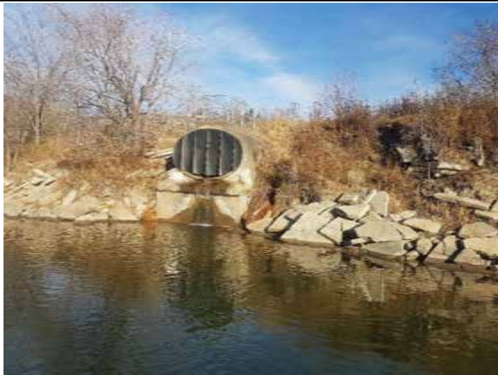
Plate 25: Looking at the Groat Ravine outfall and adjacent riprap at Government House Park.
