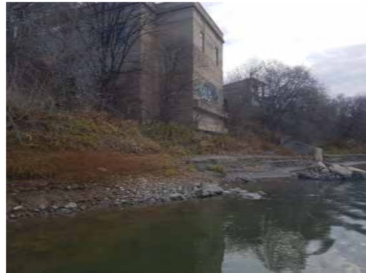
Plate 18: Looking downstream at the upstream side of Pumphouse 1 and a concrete rubble pile in the water.
