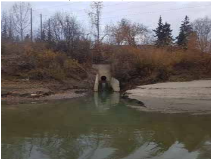
Plate 19: Looking at a functioning outfall eroding a channel in a sediment deposit between Transect 7 and 8.
