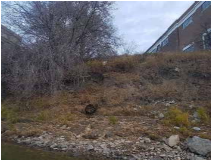
Plate 17: Looking at an outfall structure and poor riparian vegetation between Pumphouse 1 and Pumphouse 2.
