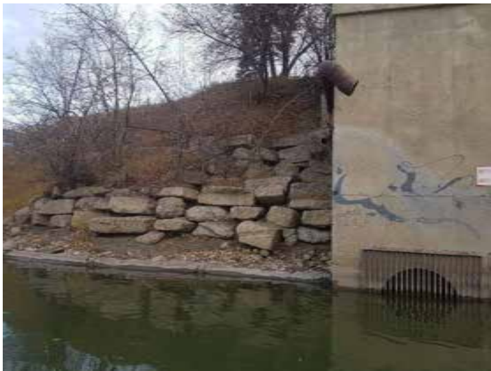
Plate 15: Looking at a concrete slab retaining wall on the upstream side of Pumphouse 2.
