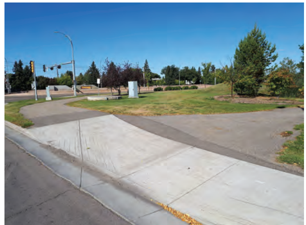
Figure 3.66: Bike Ramp from On-Street Bike Lane to Off-Street Bike Path or shared pathway
