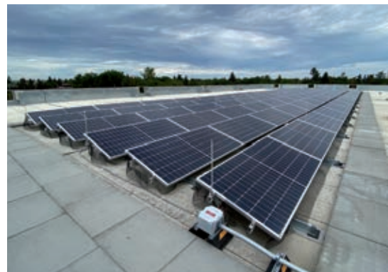
Grid-tied solar PV array
