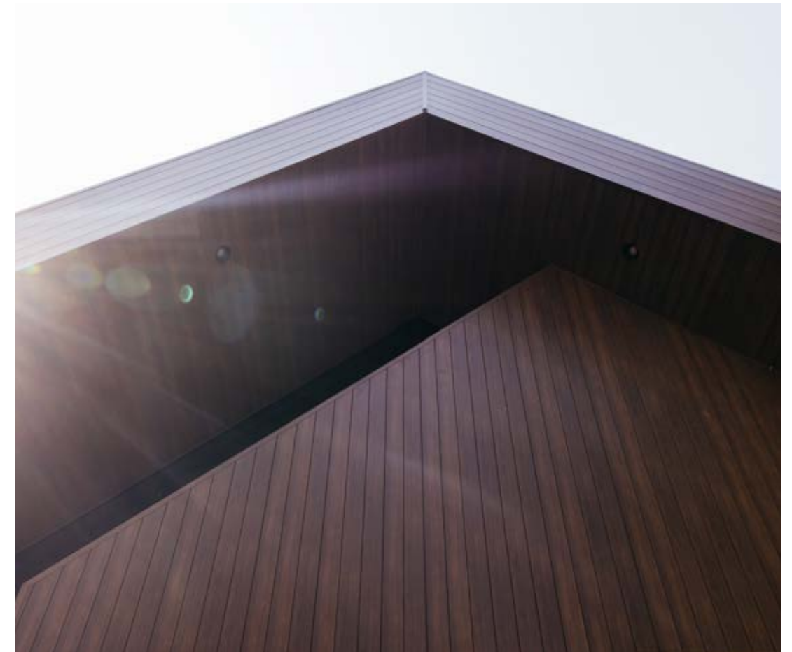
Materials used on the substation convey warmth and visual appeal, despite belonging to a utility provider.
