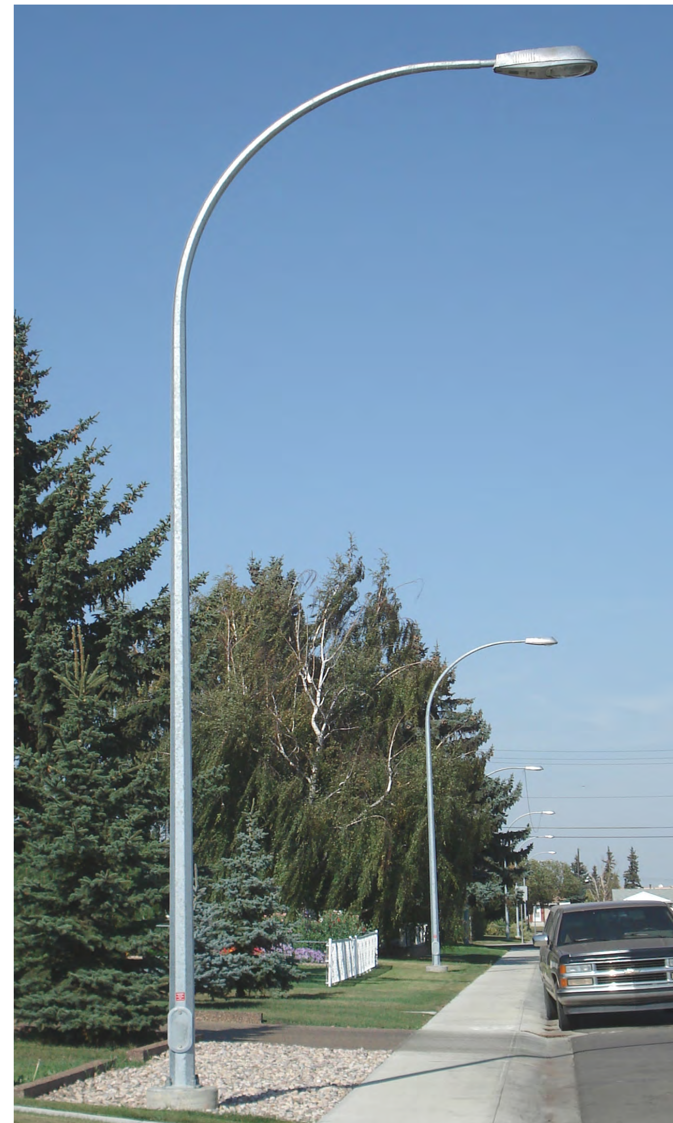
Galvanized street lights
