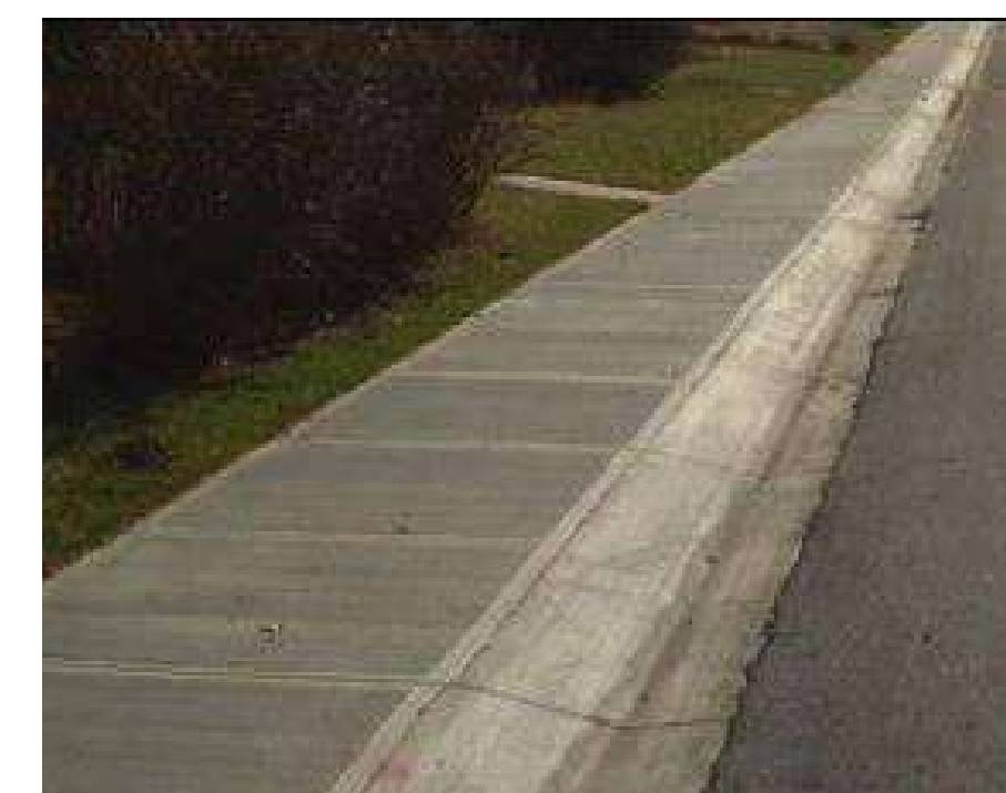
New Rolled Face Curb
