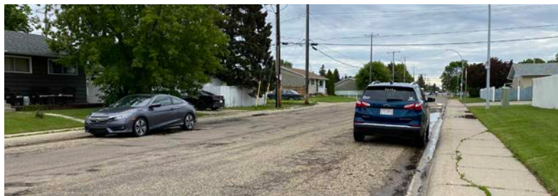
Cracked sidewalk along 165 Street
