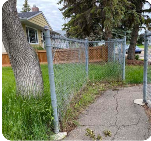
Poor accessibility due to fence
