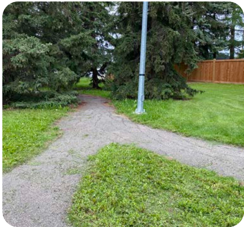
Pathway requiring upgrades
