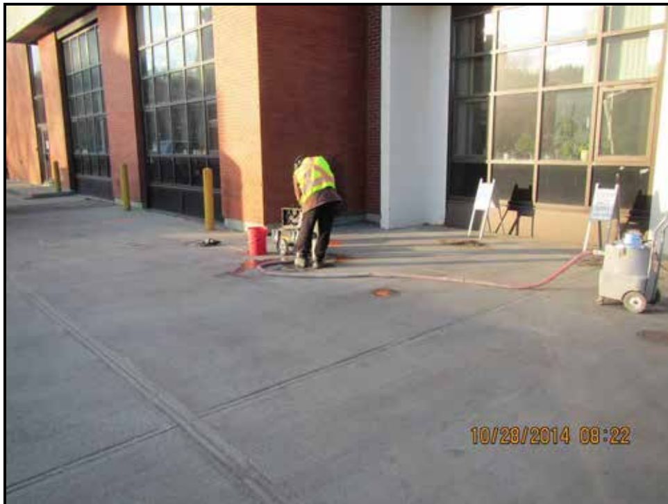
Photograph 8: Concrete coring for access to boreholes to the east of the Watermark Building within Area 7, looking southwest.
