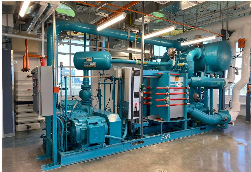
A highly energy-efficient heat pump in the Energy Centre transfers the heat from the geoexchange field to the piping that runs to the community's homes.
