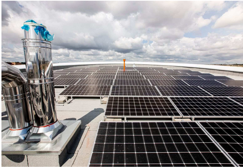
Solar panels on the roof of the Energy Centre provide renewable energy to the system.
